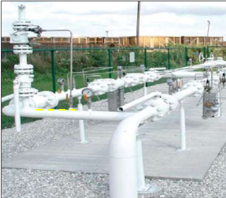
Meter and Regulator Runs
