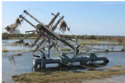
Pipeline manifold impacted by flooding
